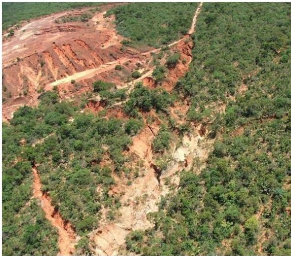
Figure 4: Destabilization of slopes downstream of the sandpit SóbritaMineração, in Serra Velha. The gully formed drains the sediment inflow into the Tigre River. Geographic coordinates UTM 23S 0621702/8125467 (43 ° 51'27 "W/16 ° 57'6" S). Source: SOUZA JÚNIOR et al. 2009, p. 7.
